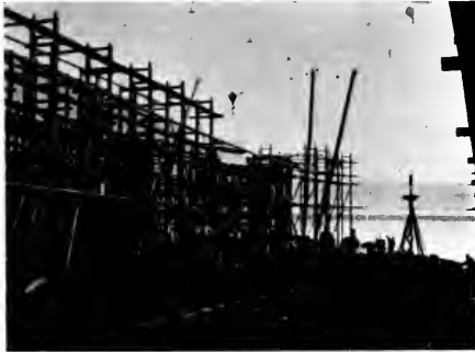
At work on one of the first big steel hulls at J. F. Duthie and Company's plant.
